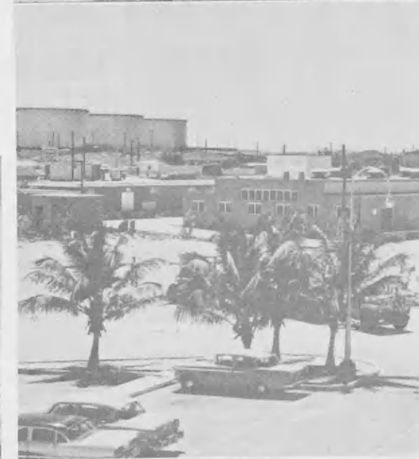
ERECTED ELEVEN years ago as a temporary h for TSD-EIG personnel was this steel-frame struct top. After relocating lab equipment and furniture, building was dismantled and moved to the barge where it was re-erected for Storehouse use. EIG personnel moved to new Administration Building offices.
